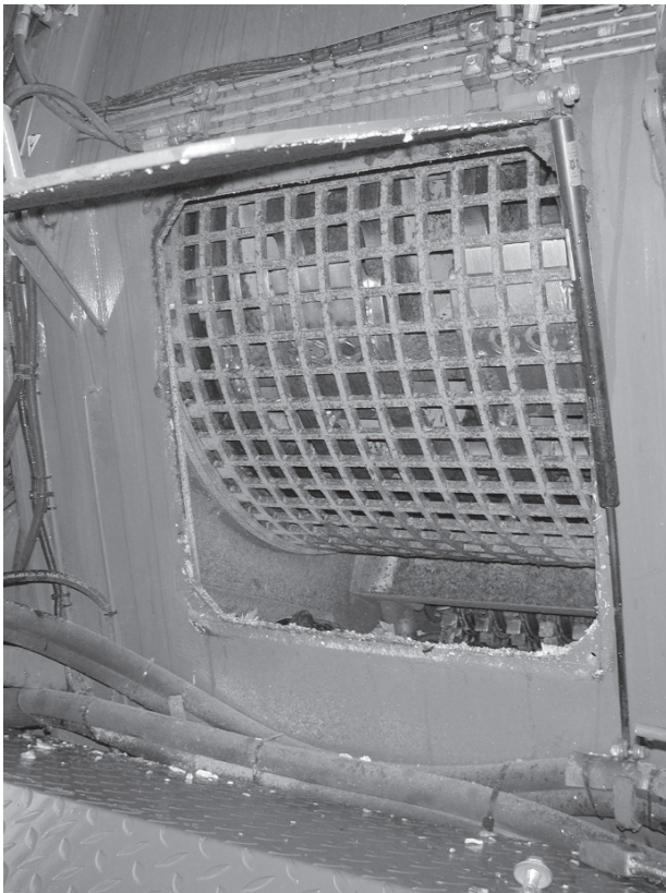
Fig. 2 The screen placed at drum case outlet
